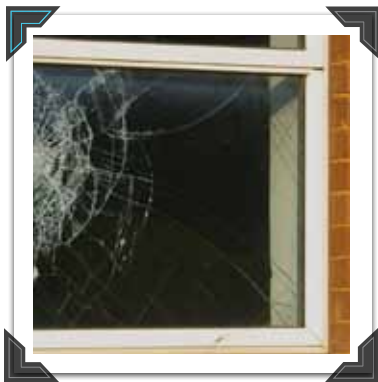
The front window gets bumped and accidentally broken.
